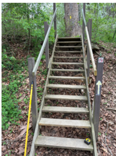
Old Stairs, supported by handrail posts with eroding footers
