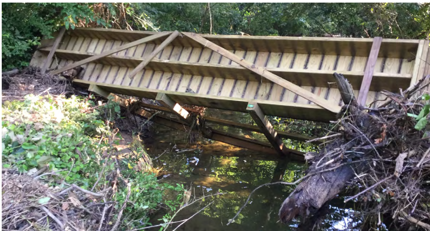
Footbridge behind the mansion relocated by flooding
